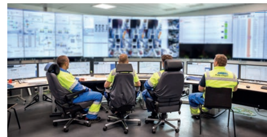
ANDRITZ supplied the Decision Support Wall (DSW) at the woodyard control room, which aids operators and maintenance groups in their daily work. It also acts as a common online remote meeting place for ANDRITZ and the operators.
