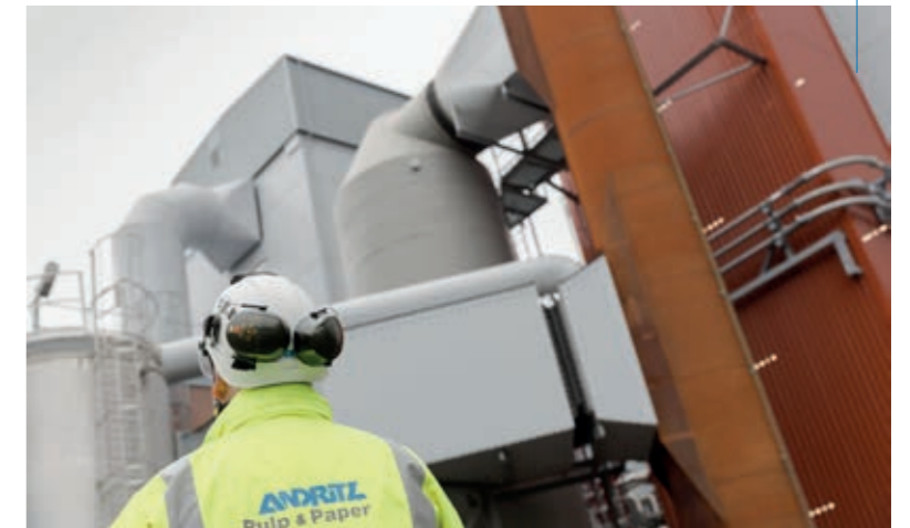
The ANDRITZ flue gas cleaning system consists of ESP, a TurboSorp system (semi-dry flue gas cleaning system), a bagfilter, and flue gas condensation. The TurboSorp plant separates the acidic components from the flue gas.
