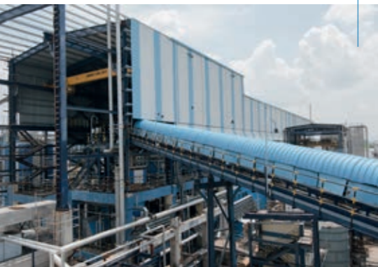
Conveyor feeding chips into the mill.
