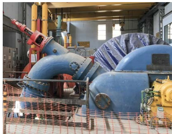
Detail of the damaged powerhouse
