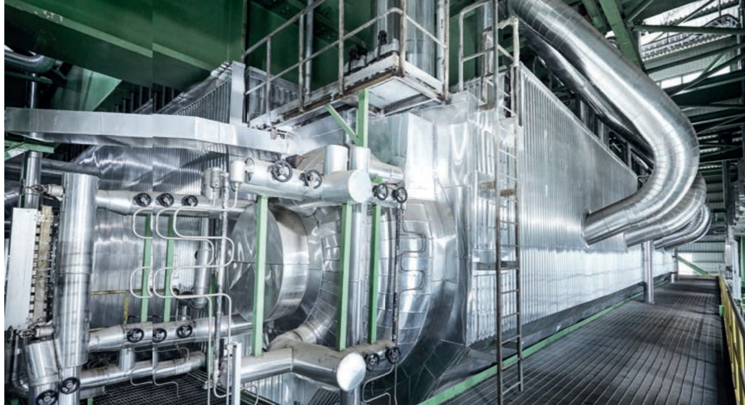
The steam drum in the OKI recovery boiler is the largest in operation today. It weighs 270 tonnes with a length of 23 m.
