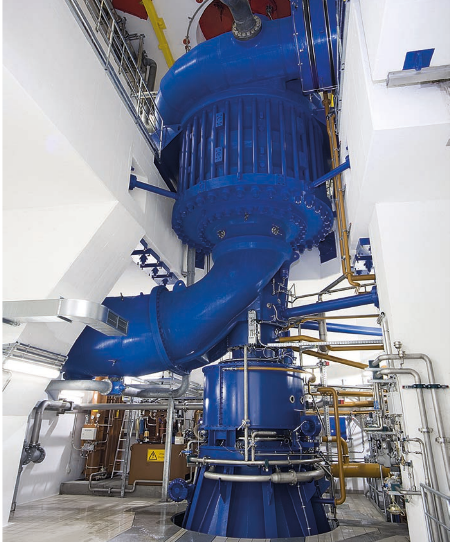
Pump turbine unit with four stages
