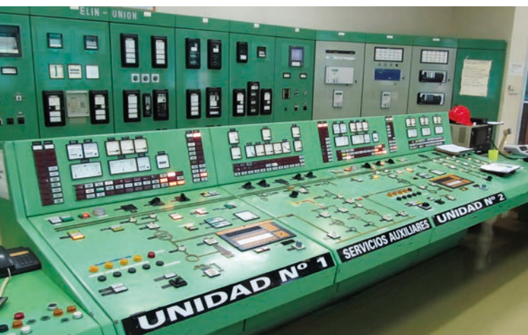
Old existing control system at HPP Carlos Fonseca
