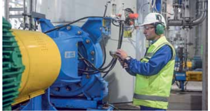
ANDRITZ delivered all the process pumps to the Montes del Plata mill. Shown here is ANDRITZ Robert Prugger, a Technician for ANDRITZ HYDRO during commissioning of a fiberline pump. ▼
