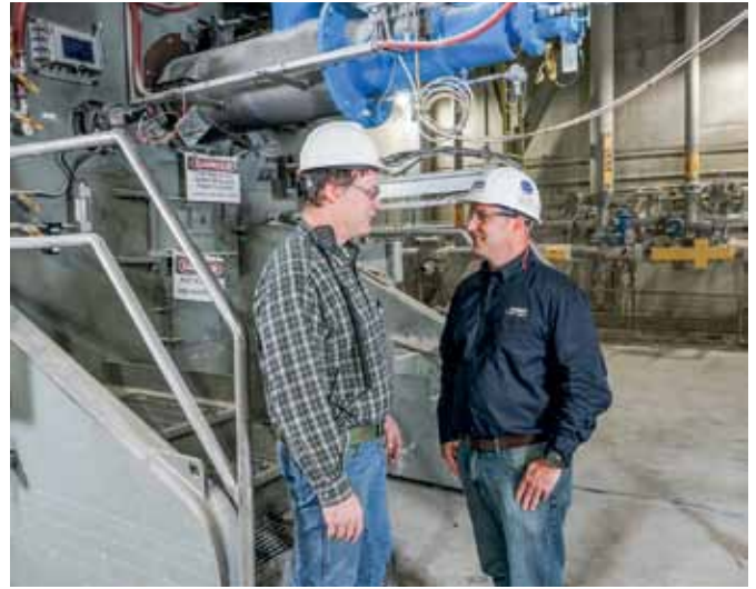
▲ Lance Bolduc, Recovery Manager (left), is shown with Todd Lewick, Burner Project Manager for ANDRITZ, with LimeFire burner in background.
