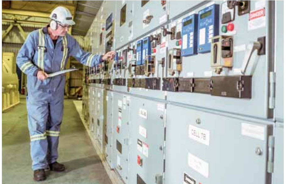
▲ Doug Tymos, Steam Plant Operator, checks the readings on a meter on the BUS-1 switchgear.
