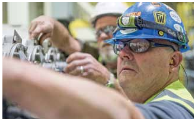
◀ Paul Goettig, ANDRITZ Commissioning Engineer adjusts an air valve for the pulse jet fabric filter.
