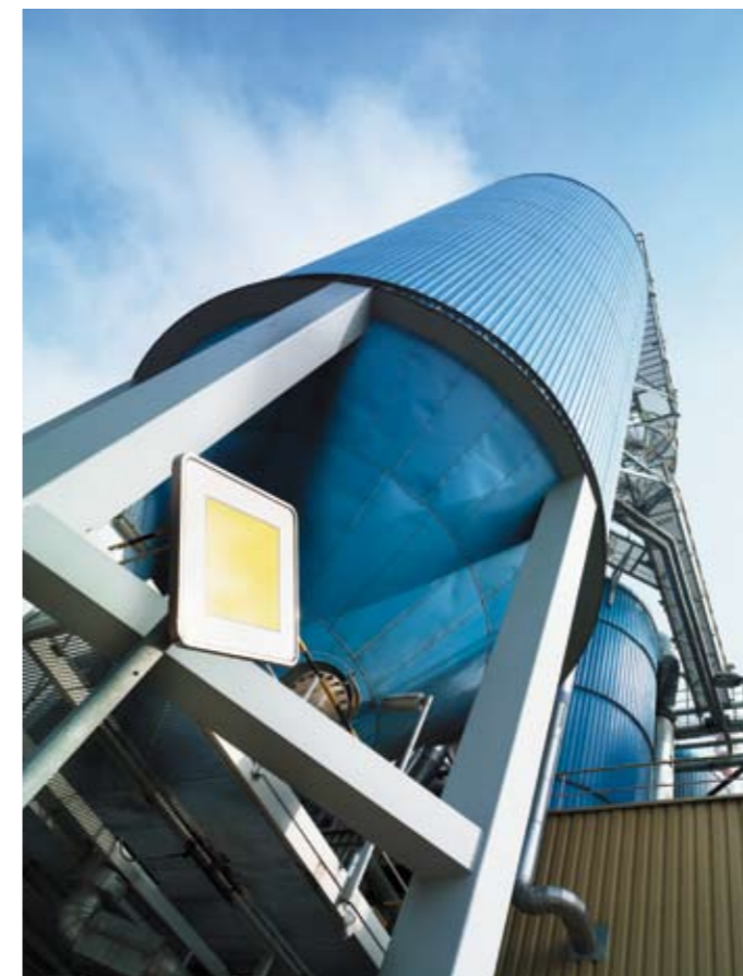
A pressurized liquor handling system, after the rebuilt 470 t/h evaporation plant, delivers 76% dry solids black liquor to the Andritz recovery boiler. The higher dry solids content of the black liquor helps lower the mill’s SO 2 emissions.
