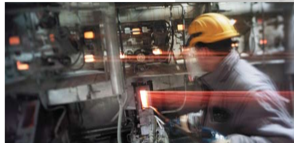
An operator cleans a liquor gun port on the firing floor of the recovery boiler.
