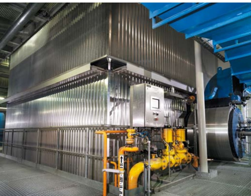
Modern natural gas load burner at the front wall of the recovery boiler.
