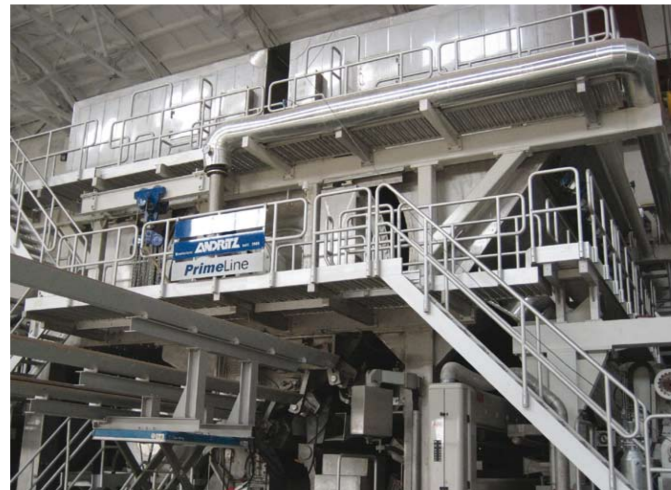
The new PM5 at Weifang City will be a duplicate of the PM3 machine shown here. It will have the capacity to produce 60,000 t/a of high quality tissue, increasing Hengan's overall capacity to over 240,000 t/a of tissue products.
