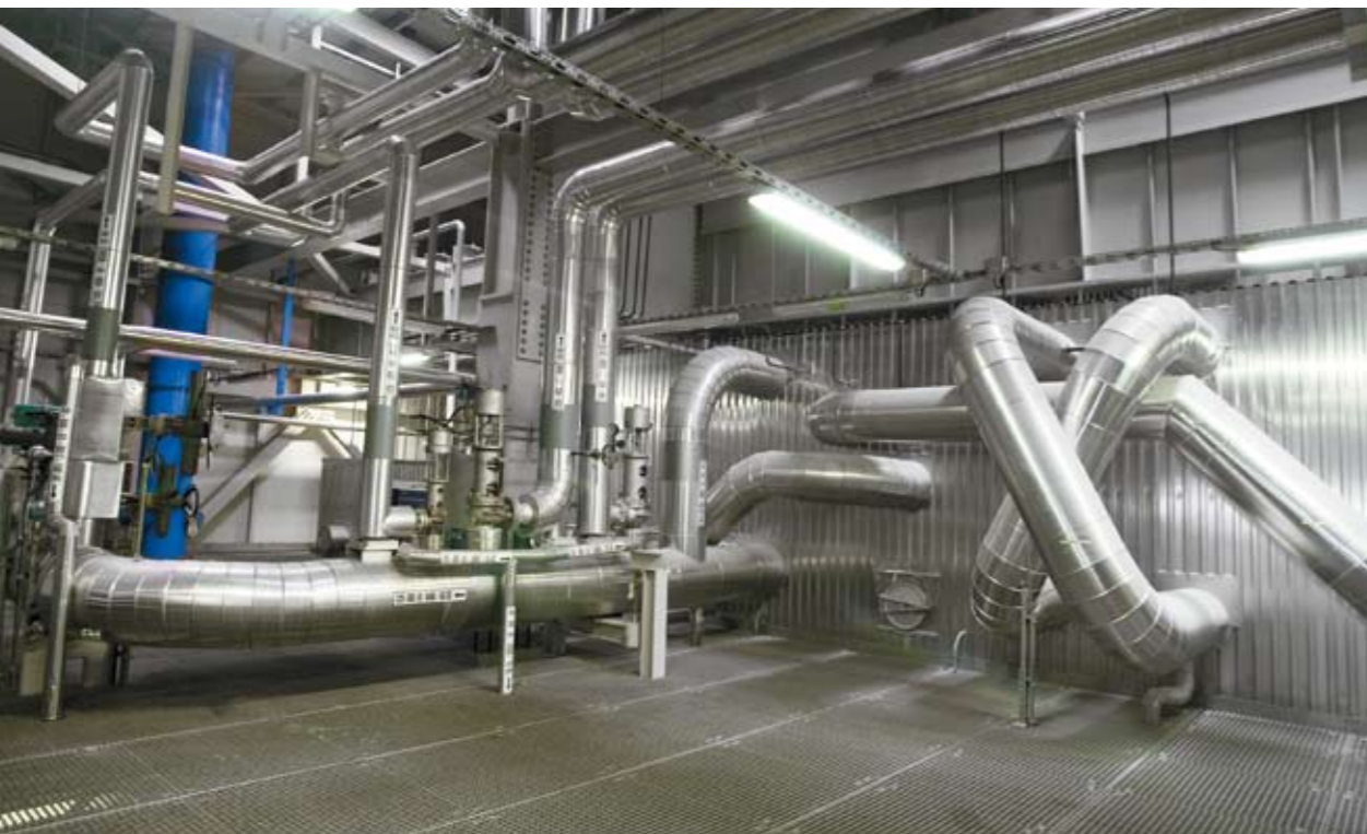
The "penthouse" of the MBP SCP's new boiler, which was delivered in only 18 months from contract signing to start-up. Shown are the main steam pipe and superheater connection pipes.
