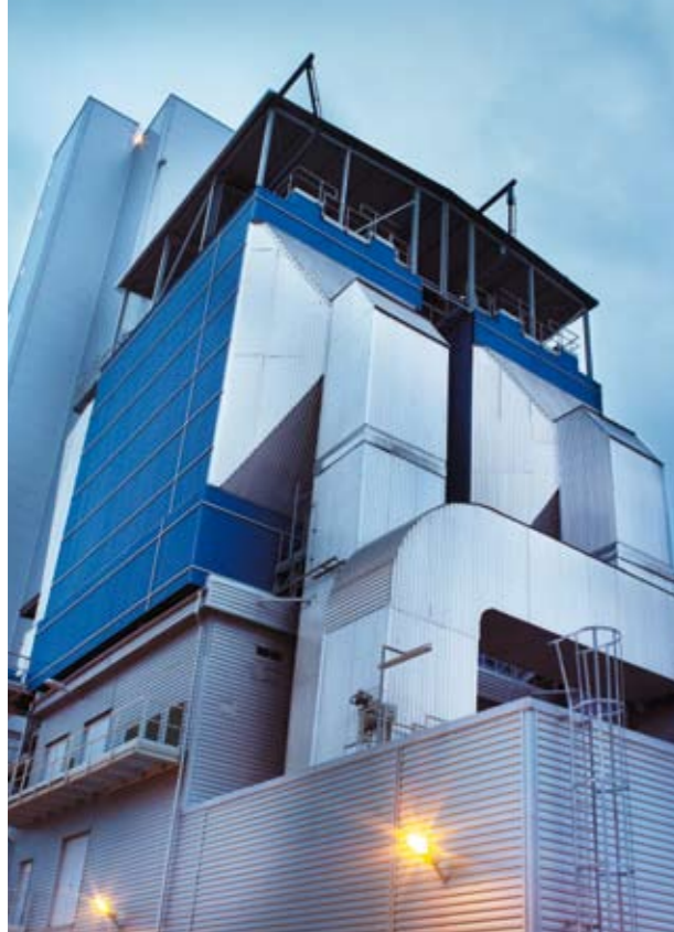
High-efficiency electrostatic precipitators contribute to the low emissions of the 900 tds/d Andritz recovery boiler.
