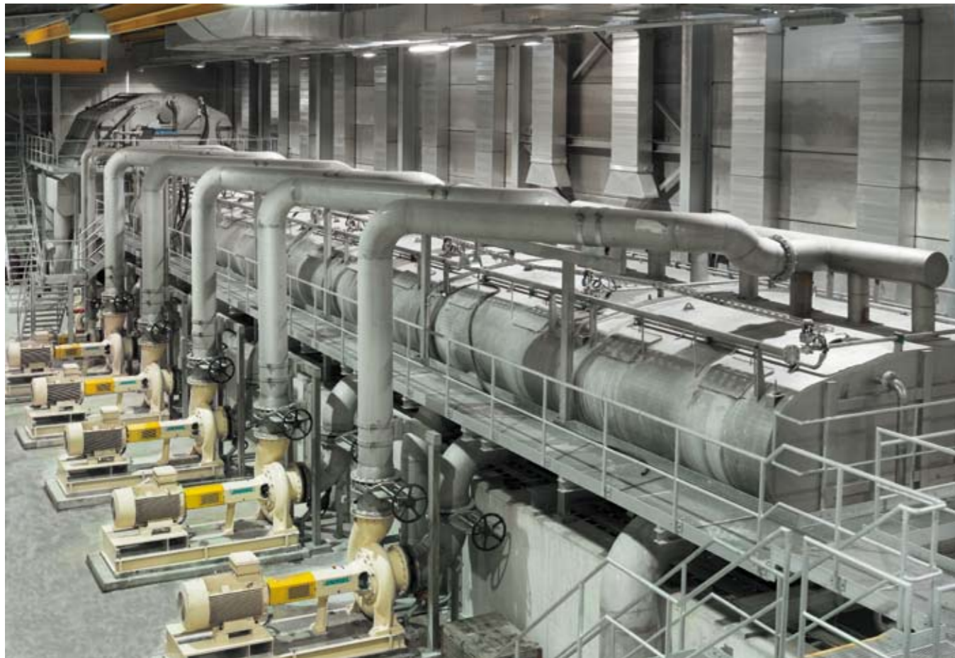
The SelectaFlot™ pre-flotation unit is the heart of the DIP process. It has six primary and two secondary cells.
